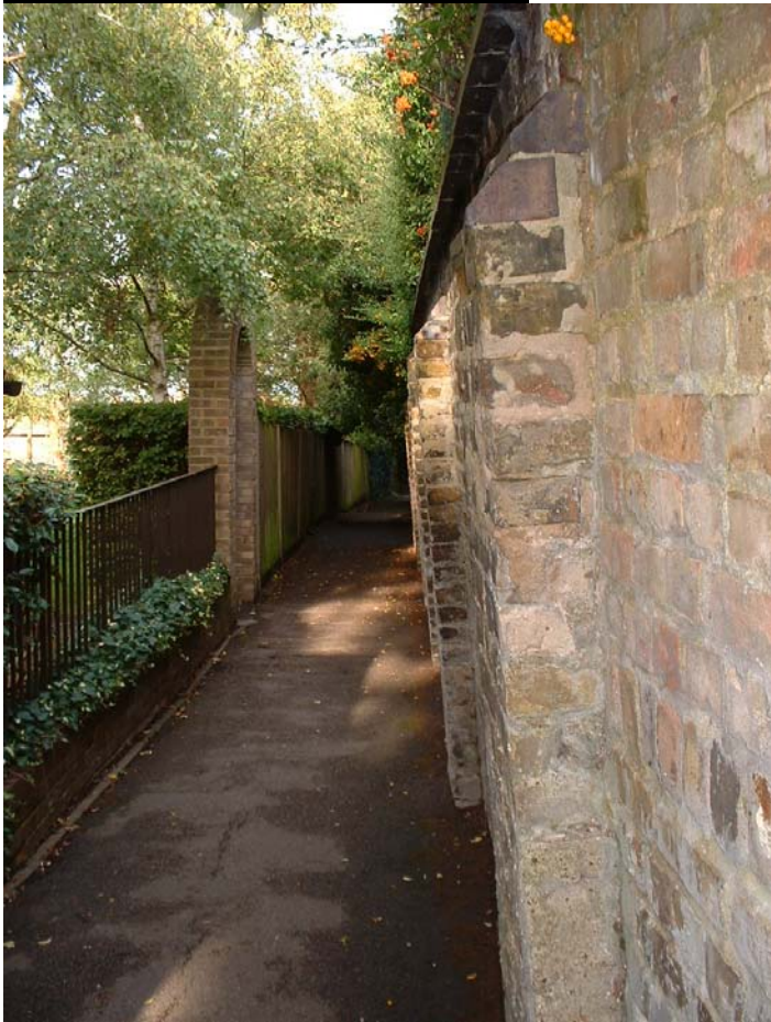
Bushey FP029 Dangerous Wall.
